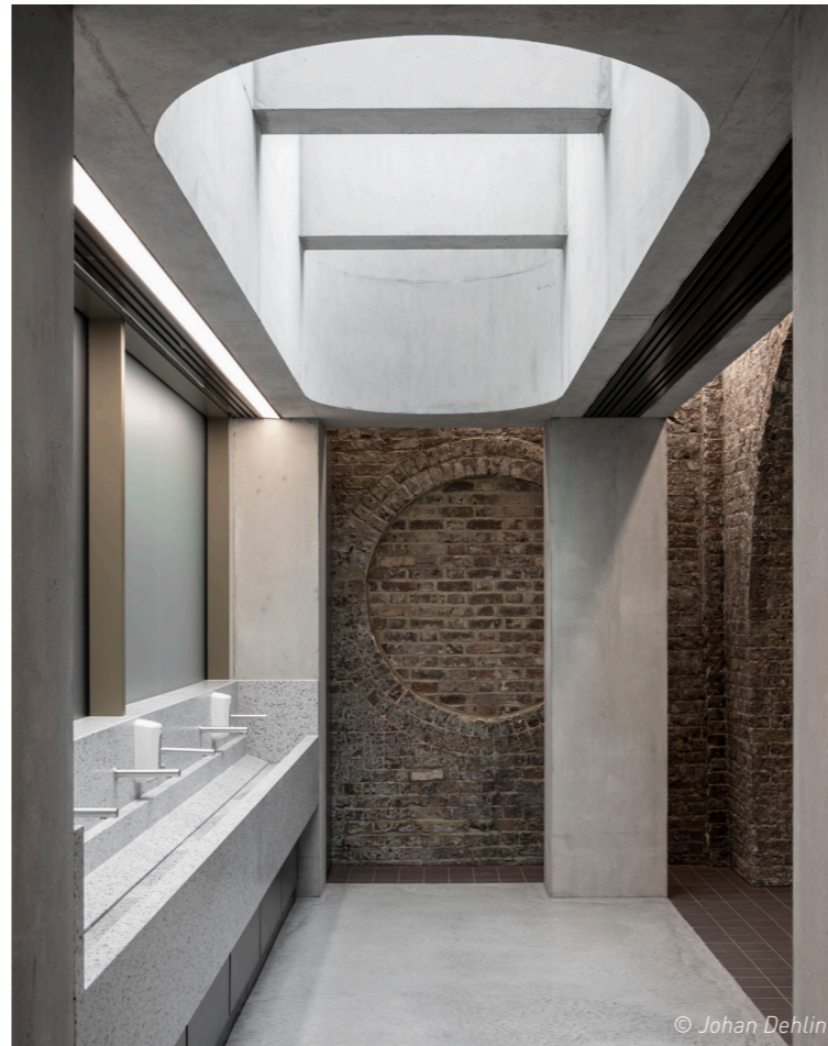
Completed WC lightwell concrete structure against existing brick wall and arch (B1)
