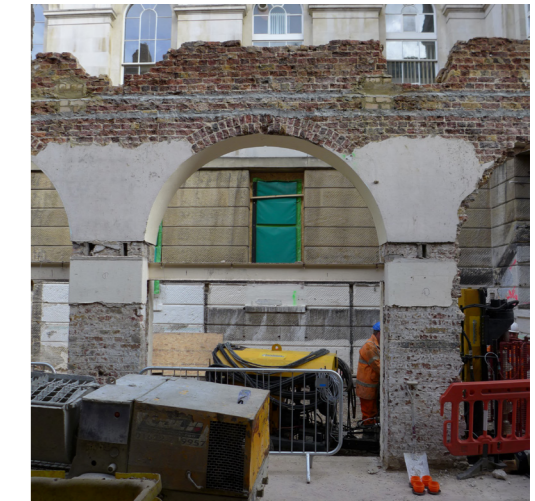
Photograph illustrating the retention of the arches, with balustrade above removed to facilitate the construction of the lightwell structures and allow for the waterproofing and insulation of the existing deck structure.
