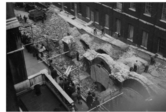
Photograph of the historic arches and vaults following WWII bomb damage, prior to the construction of the Quadrangle building in 1950s.
