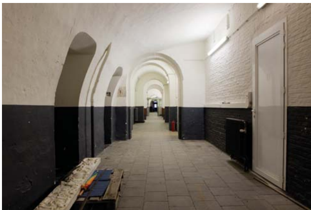
View of the situation during and after the works on the ground floor level
