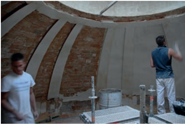
Master vault builder and plasterer working in S. Juan de la Penitencia, Alcalá de Henares, Madrid
